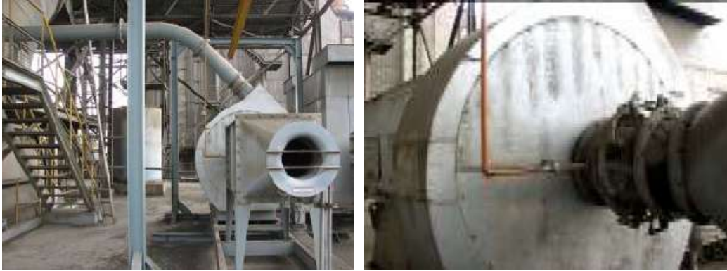
Figure 32: The ODS injection piping (left) and connection into the burner (right)
