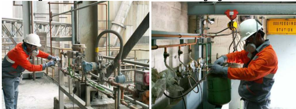
Figure 14: ODS destruction at the Holcim Narogong cement kiln
