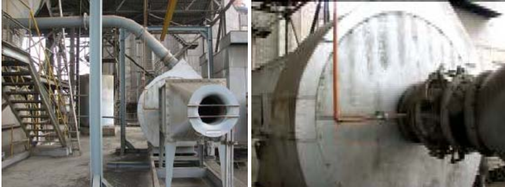
Figure 13: The ODS injection piping (left) and connection into the burner (right)
