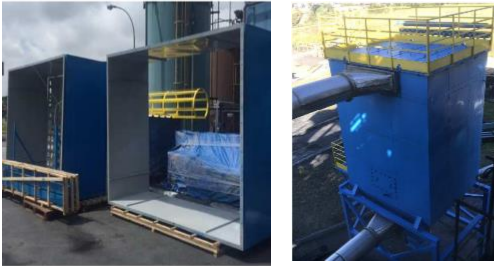
Figure 11 – Bag filter: before and after installation.
