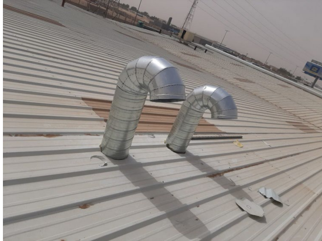
Figure 9. Exhaust vent on the roof of the production line area.
