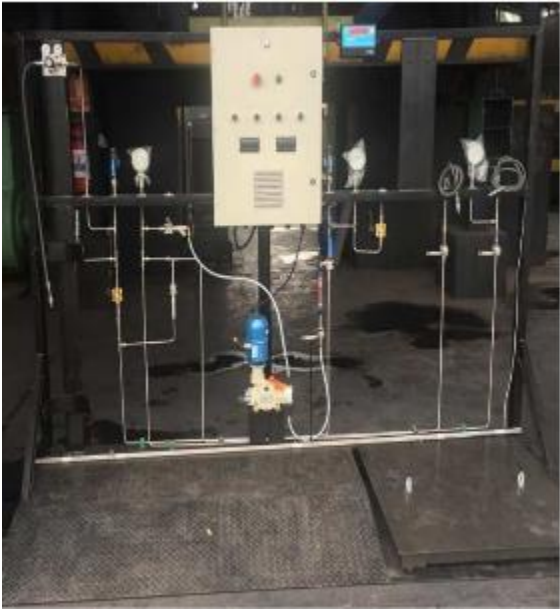
Figure 9 – Skid: Gas supply system with pressure, flow and feed weight controller.
