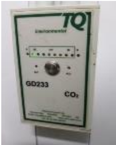
Figure 13 CO 2 Leak Detector
