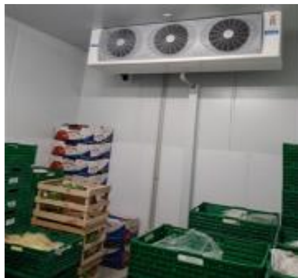
Figure 11 Walk-in Vegetable Cooler and its CO 2 Evaporator
