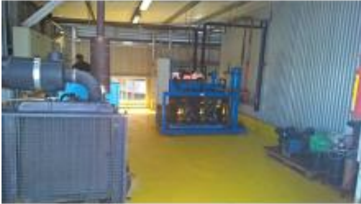
Figure 3 Baseline machine room
