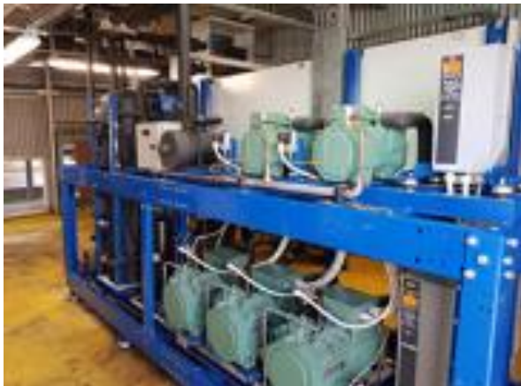
Figure 10 The CO 2 Transcritical Refrigeration Machinery
