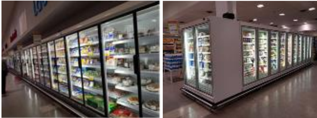
Figure 12 New CO 2 Freezer Cabinets and Aisles
