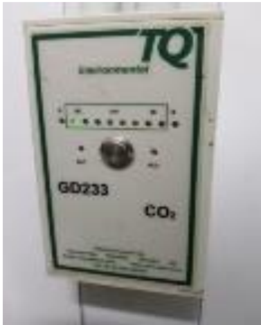
Figure 13 CO 2 Leak Detector
