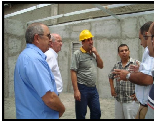
Picture 4. Project team during the construction of the ODS disposal plant. (Source: OTOZ)
