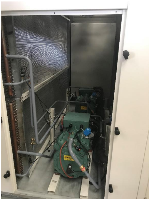
Figure 9: R-290 Unit with Semi-Hermetic Compressor
