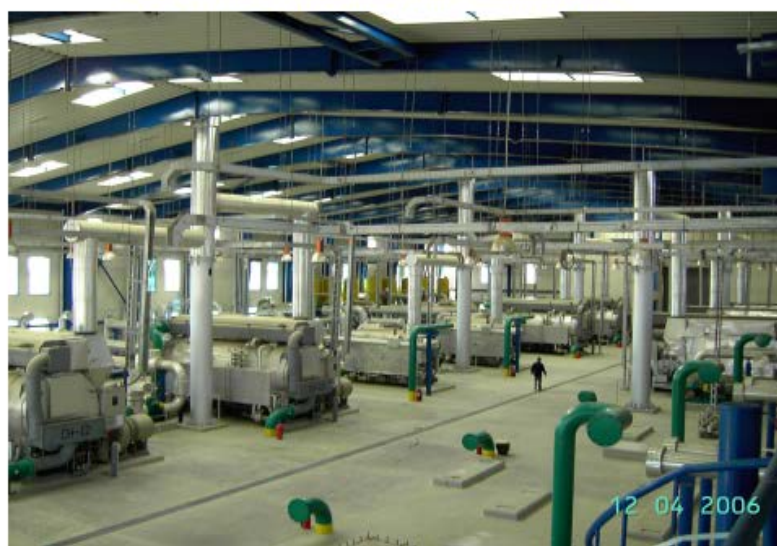
Figure 2.5: DC plant with 8000 TR gas fired absorption chiller/heaters.
