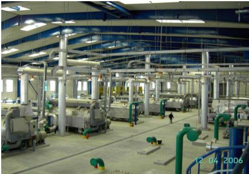
Figure 1.1: DC plant with 8000 TR gas fired absorption chiller/heaters.
