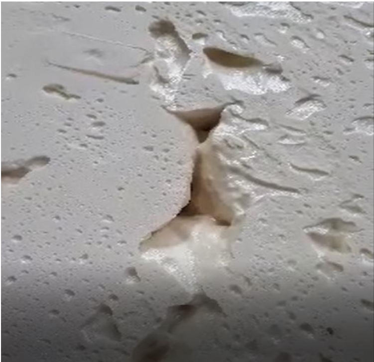
Air voids trapped inside the foam
