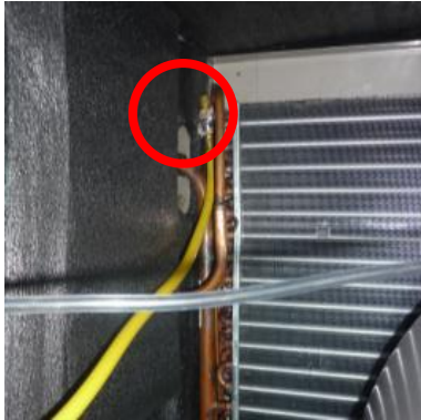
Figure 45: Leak position 1 within rooftop AHU
