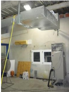
Figure 5.1: Mock elevated AHU and associated single ducting
