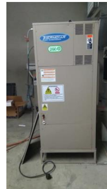
Figure 107: AHU position in test room
