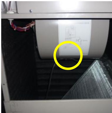
Figure 41: Sampling location #3 within ducted split AHU
