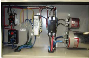
Figure 4.10: Typical contents of electrical panel
