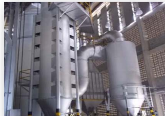
Photo 4. Quench unit and dry scrubber
