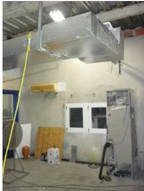
Figure 112: Mock elevated AHU and associated single ducting
