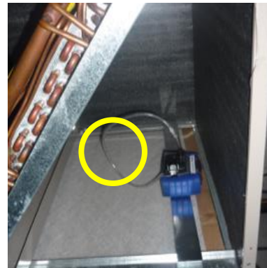
Figure 42: Sampling location #2 within ducted split AHU
