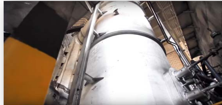
Photo 2. Secondary combustion chamber
