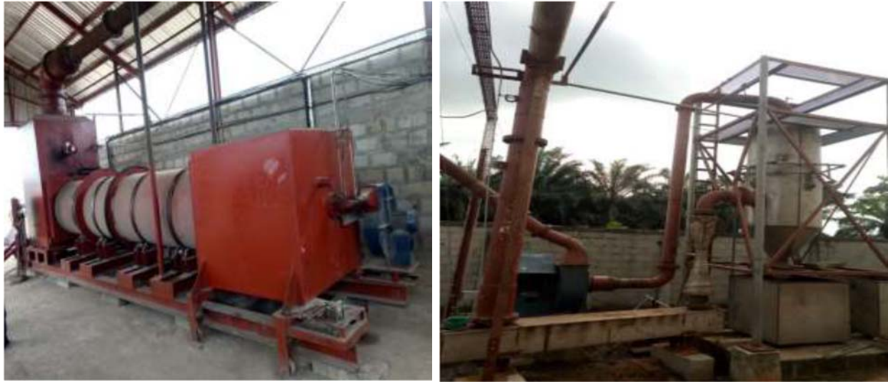
Picture 2: View of Rotary kiln incinerator and Scrubber System
