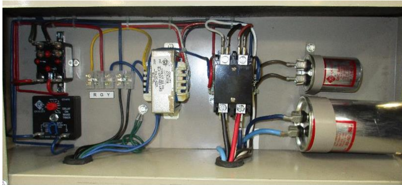
Figure 124: Typical contents of electrical panel
