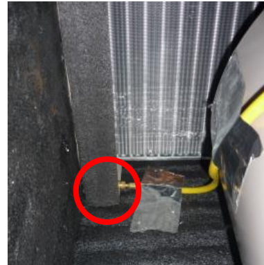
Figure 46: Leak position 2 within rooftop AHU
