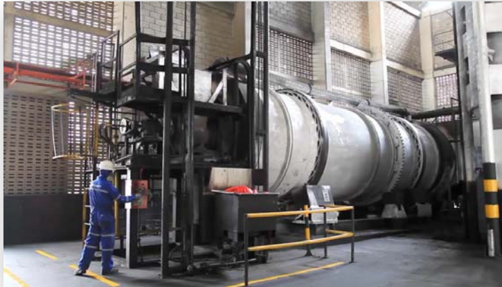
Photo 1. Primary combustion chamber (rotary kiln)
