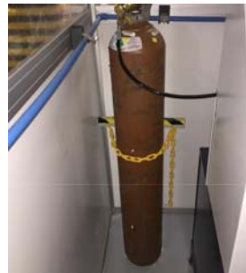
Figure 5.11: Installation of a pedestal with a safety chain to prevent the fall of the Helium cylinder.
