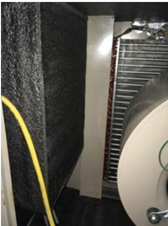
Rooftop unit release position
