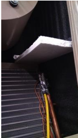
Ducted split AHU release position
