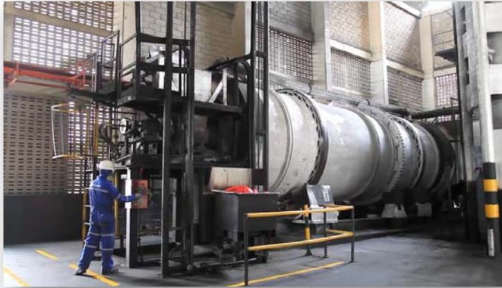
Photo 1. Primary combustion chamber (rotary kiln)
