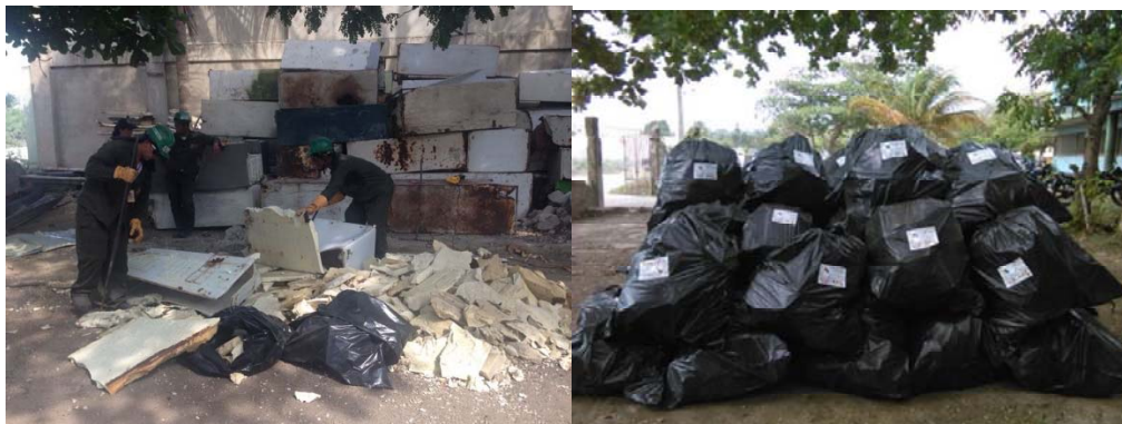
Figure 3.2: Recovery of CFC-11 based foam at San Andrés Island
