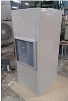
Figure 5.5: Typical contents of electrical panel
