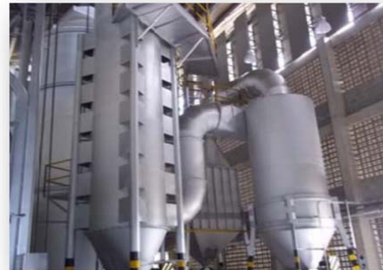
Photo 4. Quench unit and dry scrubber
