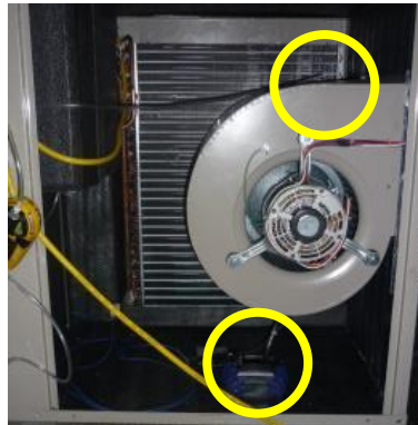
Figure 47: Sampling location #2 (base) and #3 (top) within rooftop AHU
