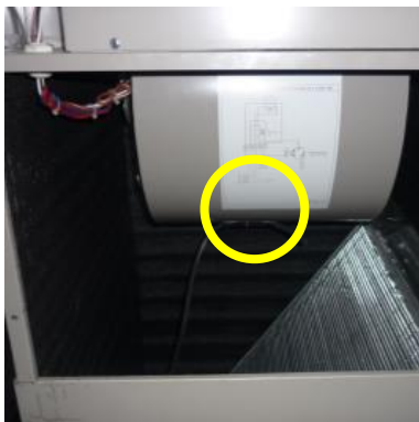
Figure 41: Sampling location #3 within ducted split AHU
