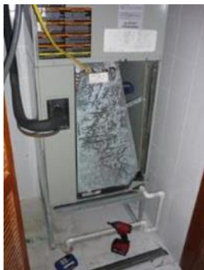
Figure 117: Ducted split AHU within closet
