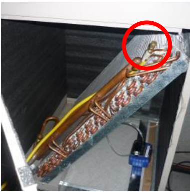
Figure 39: Leak position 1 within ducted split AHU
