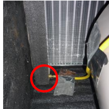
Figure 46: Leak position 2 within rooftop AHU
