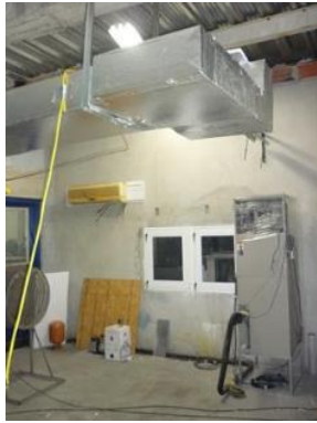
Figure 112: Mock elevated AHU and associated single ducting
