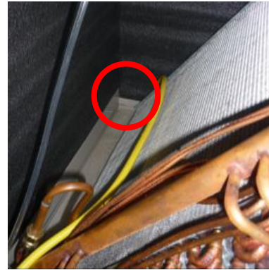
Figure 40: Leak position 2 within ducted split AHU
