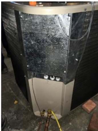
Split condensing unit electrical panel and sampling points
