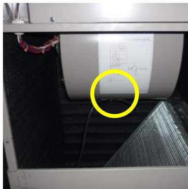
Figure 41: Sampling location #3 within ducted split AHU
