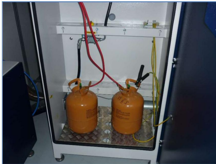
Fig. 2. R290 Cylinder Manifold
