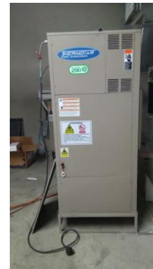
Figure 107: AHU position in test room
