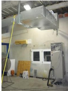
Figure 5.1: Mock elevated AHU and associated single ducting
