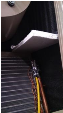
Ducted split AHU release position
