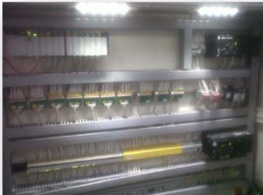
Photo 3. Automatic Control System for the combustion and post-combustion APC processes
