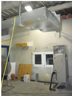
Figure 112: Mock elevated AHU and associated single ducting
