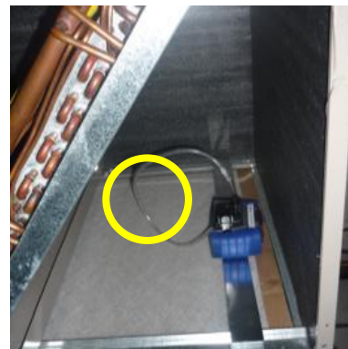
Figure 42: Sampling location #2 within ducted split AHU
