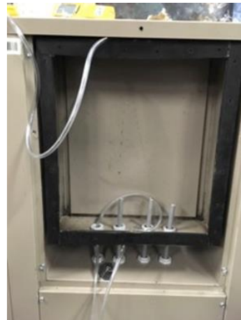
Rooftop unit electrical panel and sampling points
