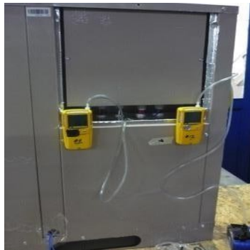
Figure 5.8: Insulated electrical box
