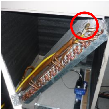
Figure 39: Leak position 1 within ducted split AHU
