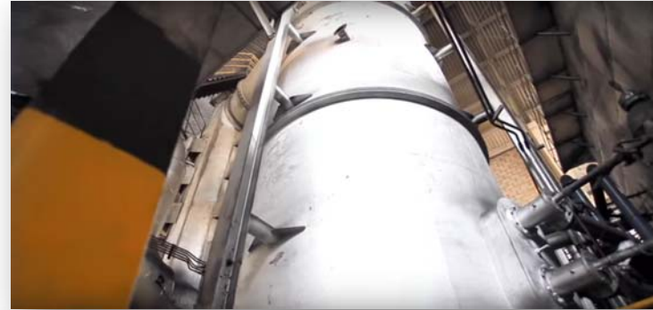
Photo 2. Secondary combustion chamber
