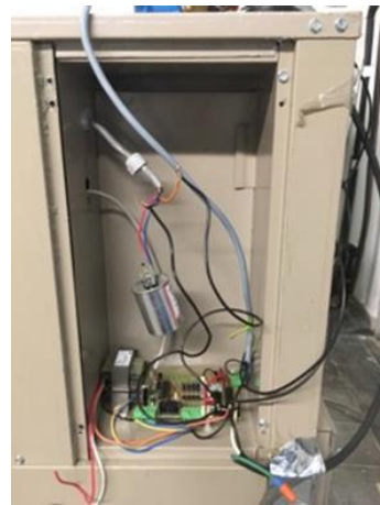
Ducted split AHT electrical panel and sampling points
