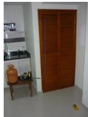
Figure 118: Closet containing ducted split AHU
