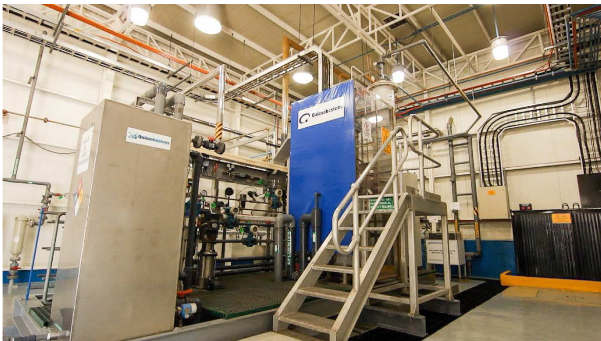
Figure 13 Argon plasma arc at Quimobásicos facilities in Monterrey, Mexico
