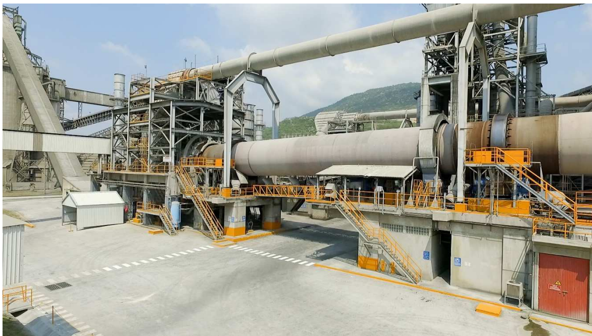
Figure 14 Cement kiln at Holcim Mexico facilities in Colima, Mexico
