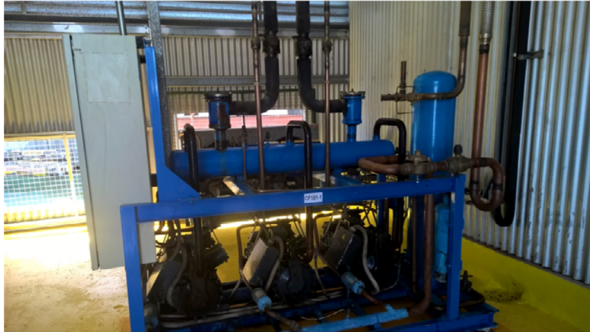
Figure 13 Medium temperature compressor pack (3 compressors)
