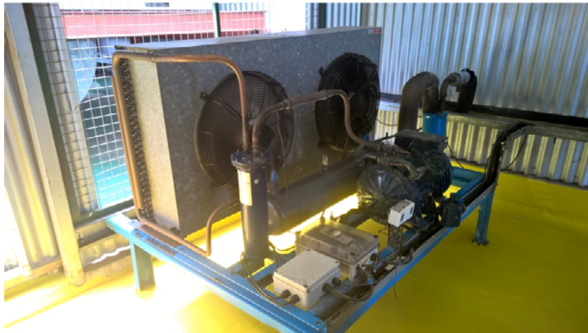
Figure 14 Low temperature compressor, condenser, receiver, oil separator
