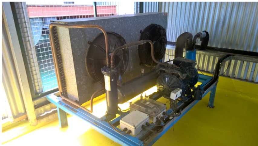
Figure 14 Low temperature compressor, condenser, receiver, oil separator
