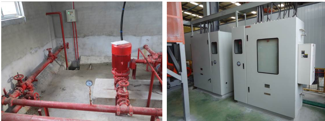
Fire equipment and anti-explosive control cabinet
