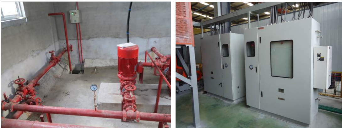
Fire equipment and anti-explosive control cabinet
