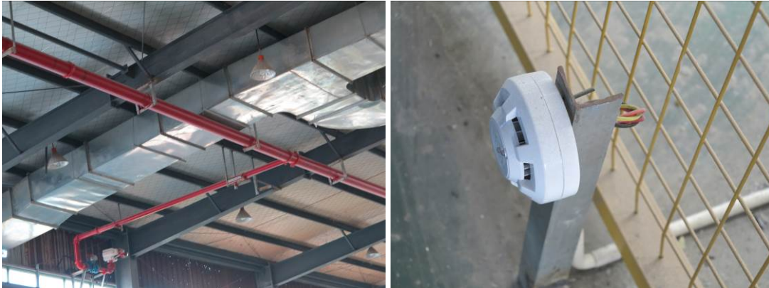
Forced ventilation system and highly sensitive flammable gas sensor
