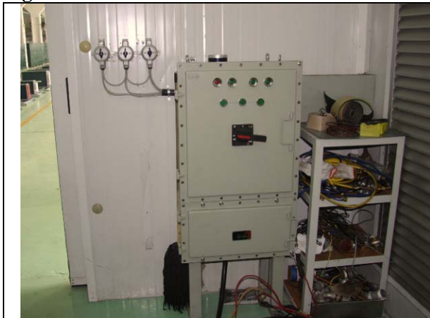
Electric explosion-proof cabinet
