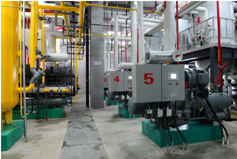
Fig 15. Running NH 3 /CO 2 system in customer
