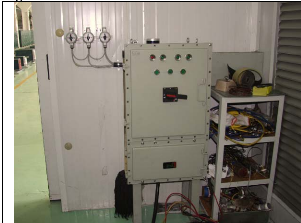
Electric explosion-proof cabinet
