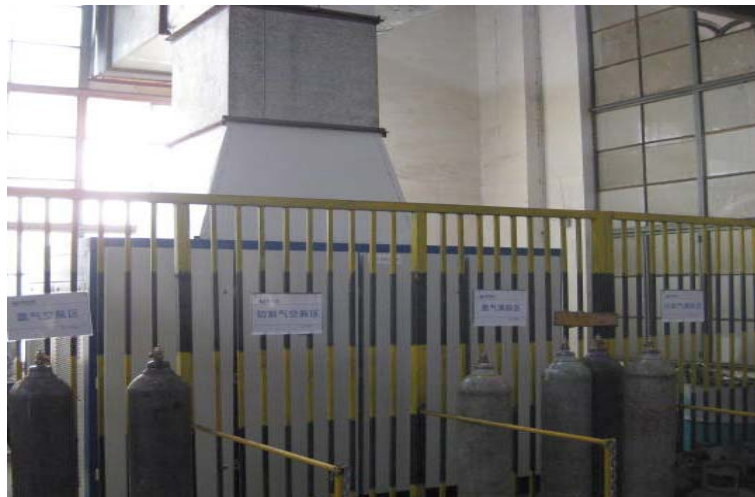
Fig 9. High pressure test equipment for CO2 vessel
