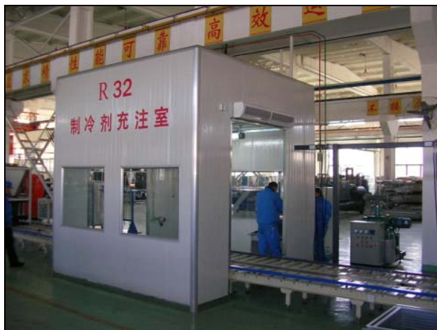
R32 charging room
